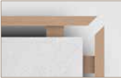
open miter joint
