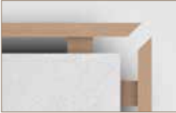
open miter joint
